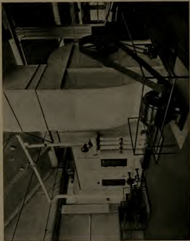
Planooidal Type "L" Fan and Heater Installed with Humidifier
